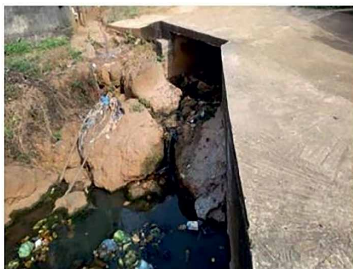
Figure 17. Gutters discharging wastewater and toilet water into the lake.
