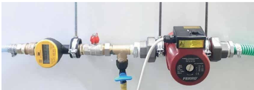
Figure 8. Components of the water circuit, which ensure the circulation of the flow captured through the water intake model.
