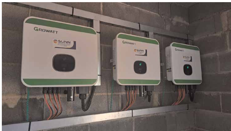
Figure 2. Inverter applies at plant for doing grid zero. Source: Author himself.
