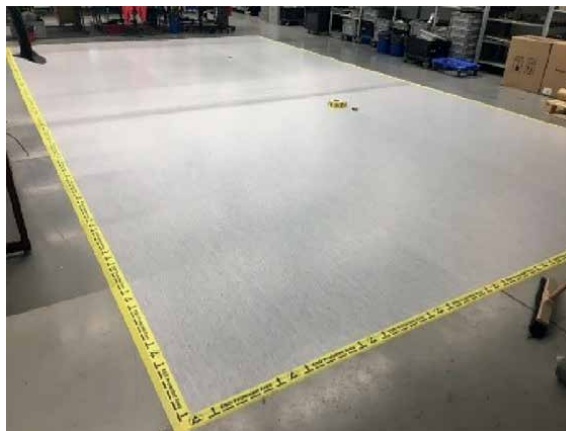
Figure 6. Bonded ESD flooring in PVC design with floor EPA marking.
