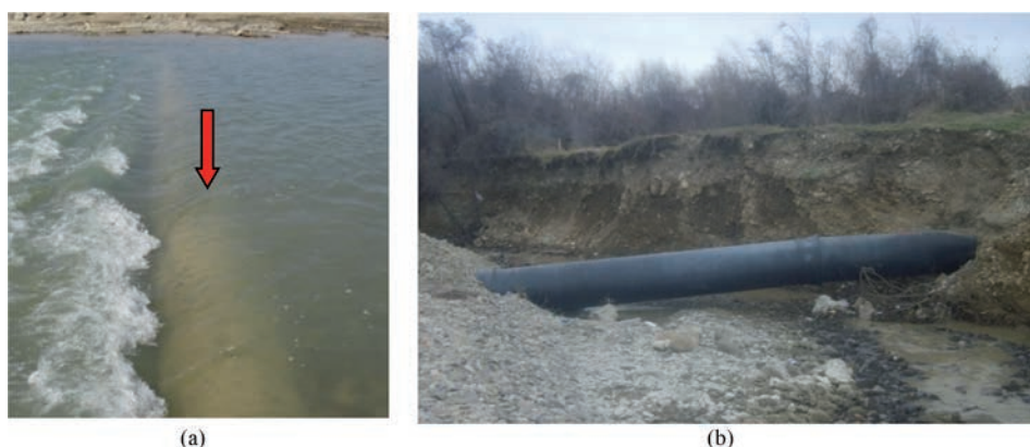
Figure 4. Pipes located in the undercrossing of a river bed uncovered by the action of a series of floods with high flows: a – the supply pipe with D = 1000 mm on the Moldova River [19]; b – the supply pipe with D = 800 mm on the Tazlaul Sarat River [20].
