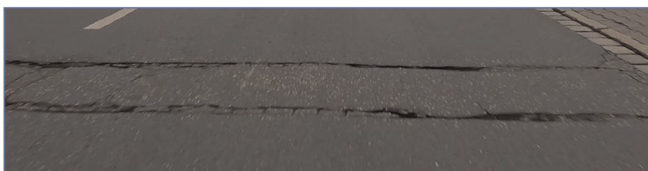
Figure 3. Road damage at maximum acceleration deflection [5].
