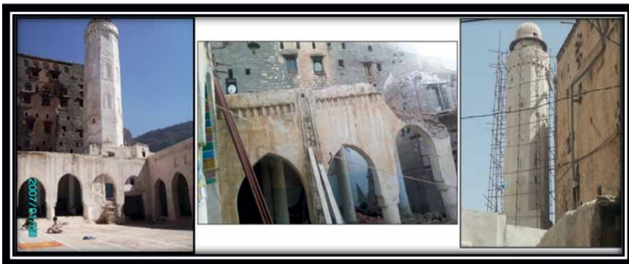
Figure 18. Omer bin Al Khattab Mosque's collapsed minaret.
