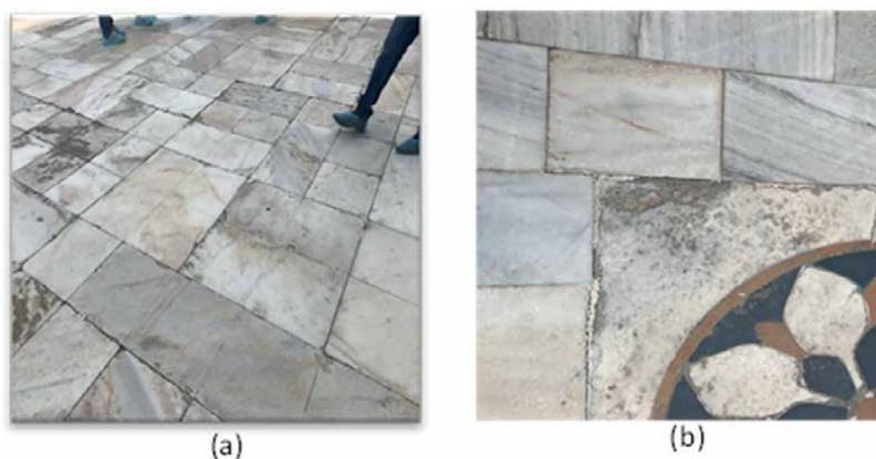
Figure 3. (a) Pitting and uneven surface observed on the exterior floor slab of the Taj Mahal. (b) Pitting and uneven surface observed on the exterior floor slab of the Jaswant Thada.
