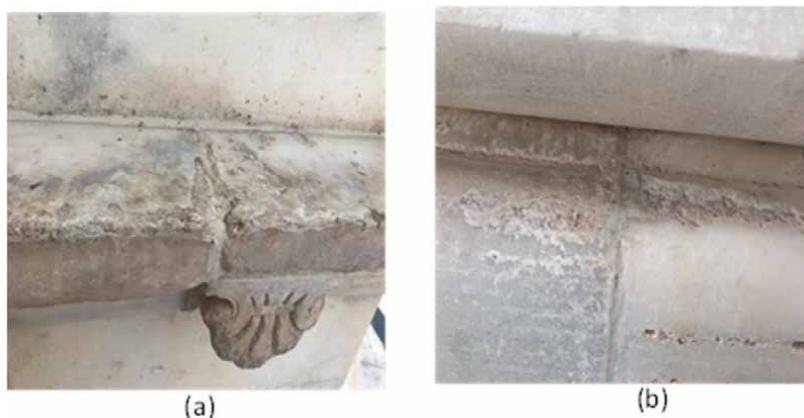
Figure 2. (a) Spalling and disintegration observed on the horizontal slab placed on the exterior wall of the Jaswant Thada. (b) Spalling and disintegration seen on the exterior walls of the Jaswant Thada.
