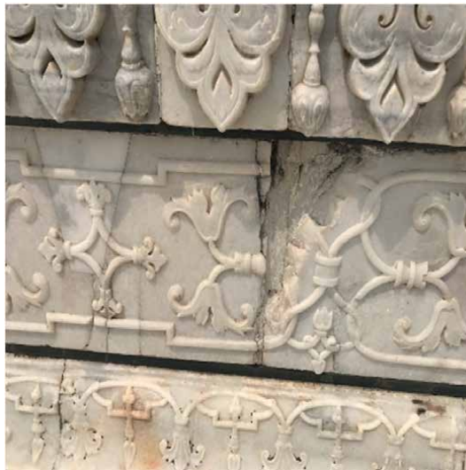
Figure 10. Cracks observed on the intricately designed vertical marble slabs placed on the base (a platform for the main mausoleum of the Taj Mahal).
