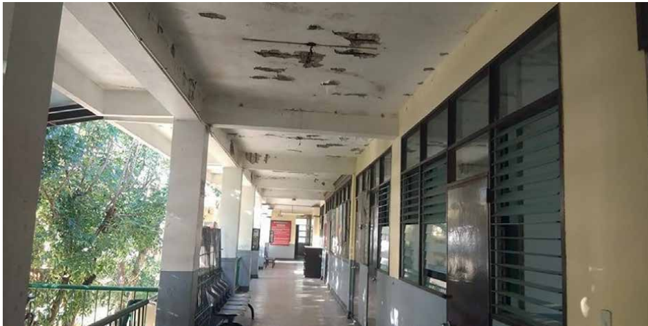
Figure 11. Federizo Hall—third floor ceiling with visible severe damaged due to age.
