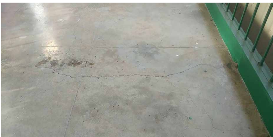
Figure 12. Federizo Hall—third floor slab with visible cracks.
