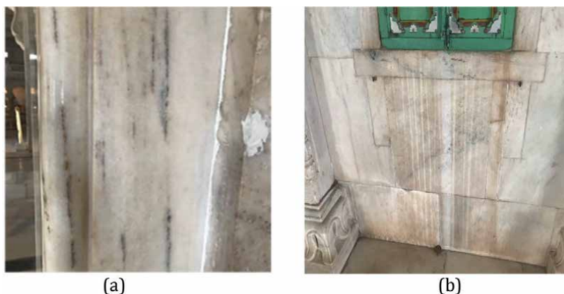
Figure 4. (a) Dark brown and black stains observed on the exterior wall on the entrance gate of the Jaswant Thada. (b) Brown stains observed below the window sills on the exterior walls on the Jaswant Thada.
