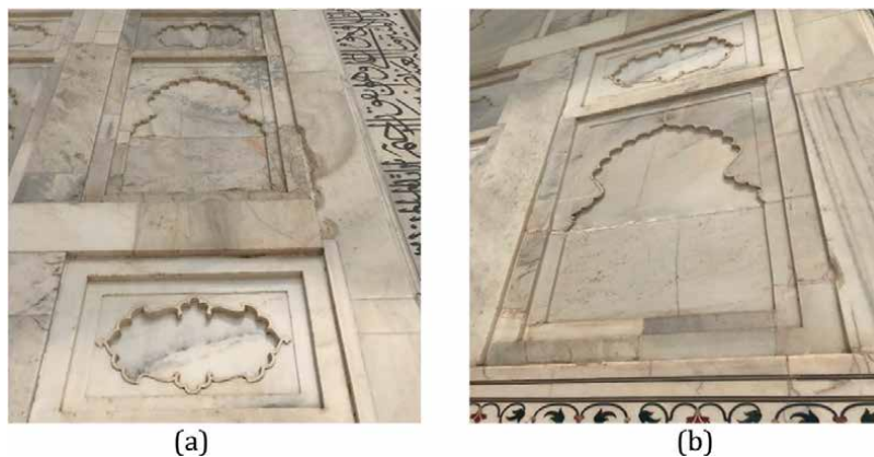
Figure 11. (a) Different crack patterns on the exterior walls of the Taj Mahal (b) Vertical crack patterns on the exterior walls of the Taj Mahal.
