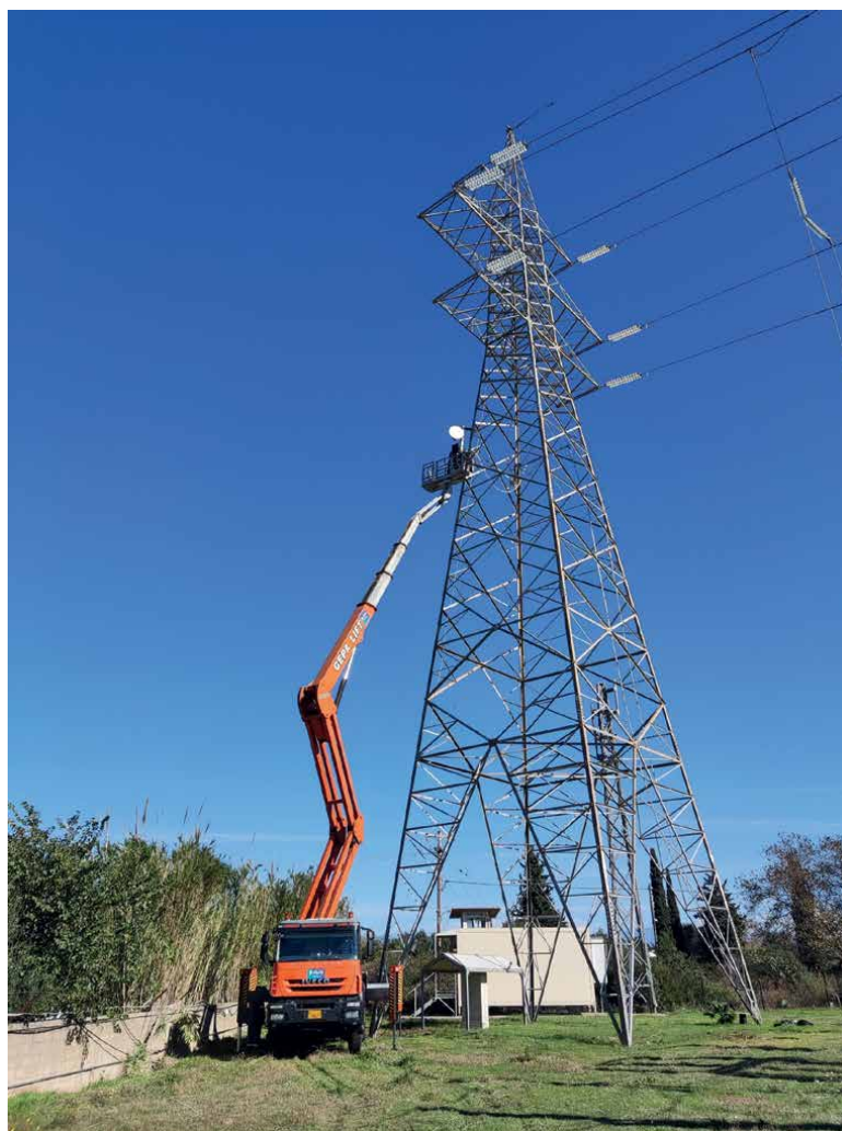
Figure 7. Installation of mmWave antenna equipment linking ADMIE and UoP sites.
