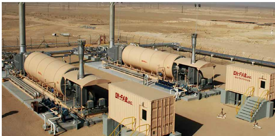
Figure 2. Conventional OTSG boiler. Source: www.en-fabinc.com .
