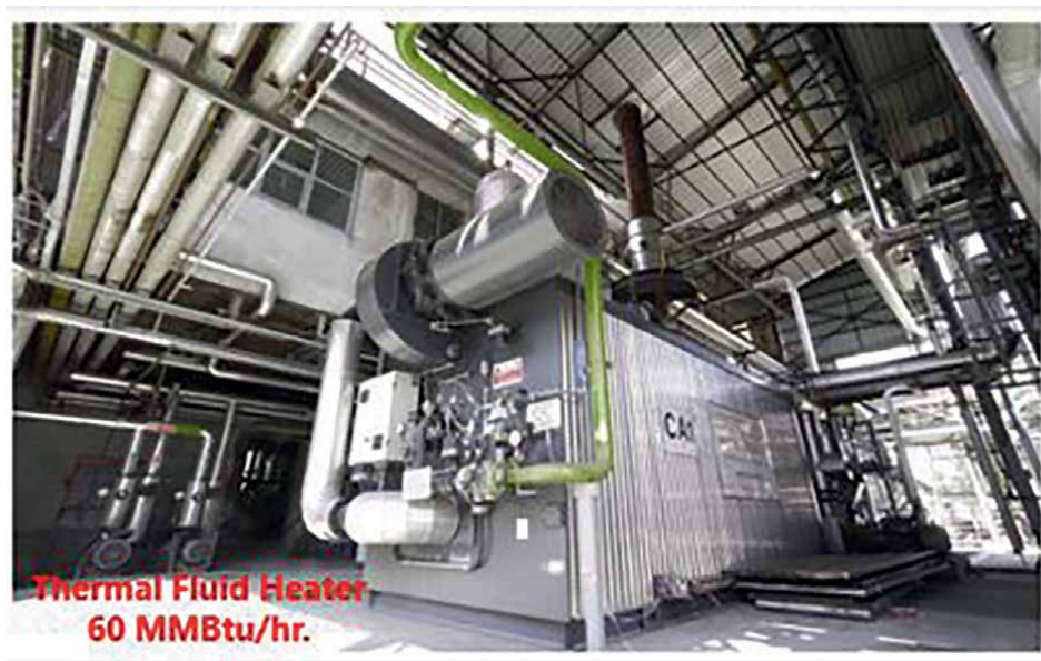
Figure 6. 60 MMBtu/hr. thermal fluid heater. Source: www.caiz.com .
