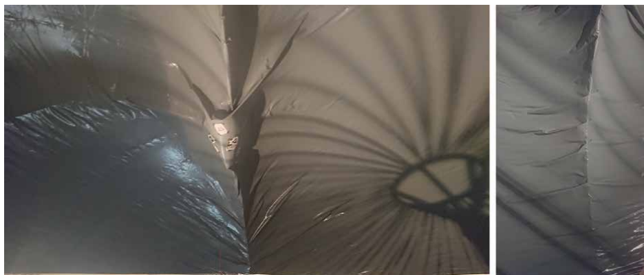
Figure 24. Folds in the gas membranes caused by measuring devices, below the gas membrane (left), from above (right) [© Kai Heinlein].
