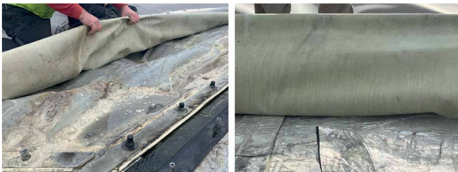
Figure 7. The sulphur is deposited on the insulation in a three-layer membrane with condensation (left) and on the inner side of the gas membrane (right) after one year in use [© Rosemarie Wagner].
