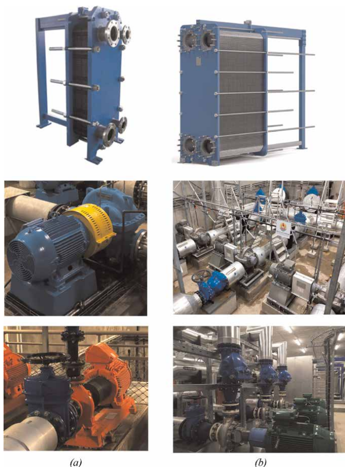
Figure 3. Plate heat exchanger, primary pump, and secondary pump for Tetiaroa (a) and Tahiti (b).
