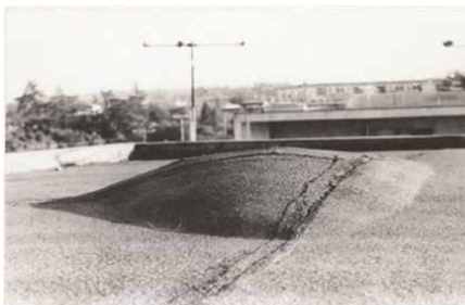
a) Swelling of waterproofing
