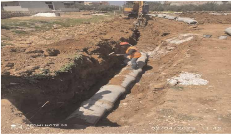
Figure 4. The buried sewerage concrete pipeline is being implemented in the town of Jabab in Dara-Syria.
