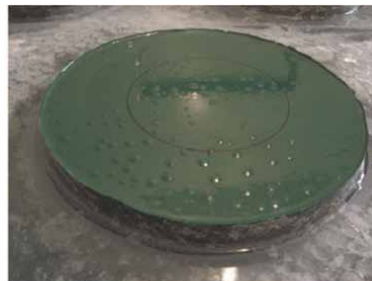
b) Blistering of floor coating
