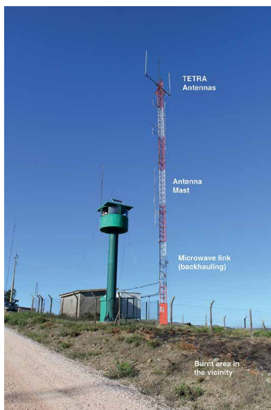
Figure 9. Illustration of Reliable Wildfire Communication: Microwave links with 1 + 1 redundancy ensure uninterrupted, resilient connectivity between communication towers, enabling seamless coordination for firefighters in critical wildfire response scenarios.
