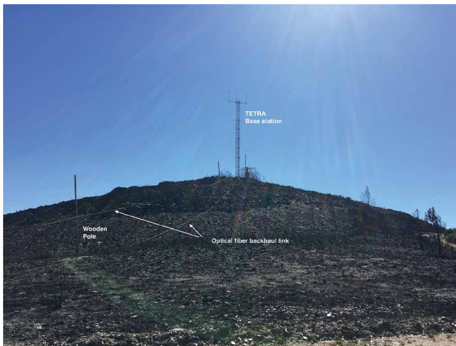
Figure 1. Single point of failure: Optical fibre backhaul link affected during a wildfire.
