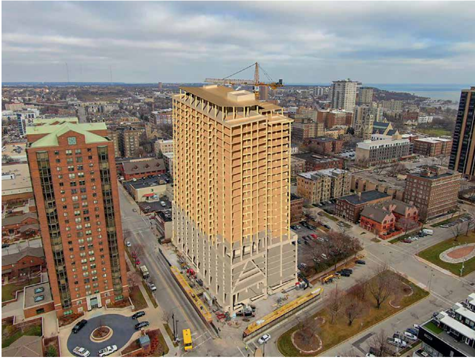
Figure 1. Photograph of the ascent MKE building under construction revealing the extensive use of mass timber products in the supporting structure [2].
