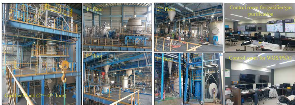
Figure 16. View of each floor and control room in demo-scale plant.
