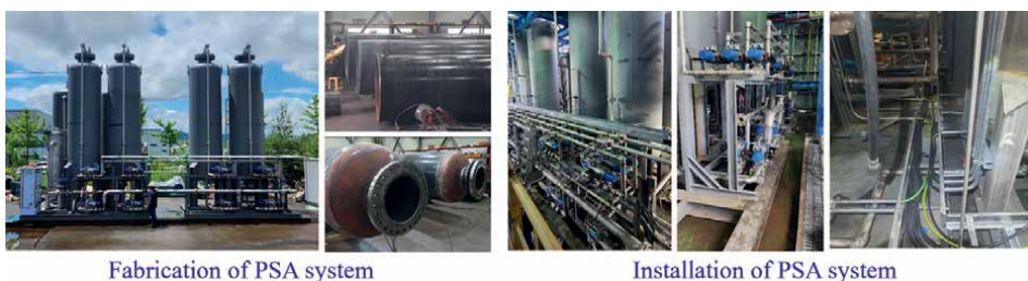
Figure A6. Fabrication and installation of PSA system (syngas treating capacity 1600 ~ 2500 Nm 3 /h) in demo-scale plant.
