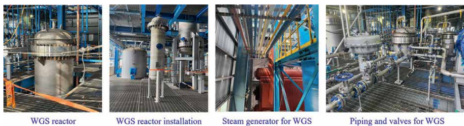
Figure A5. Key components of WGS system (syngas treating capacity 1600 ~ 2500 Nm 3 /h) in demo-scale plant.
