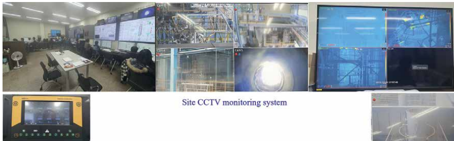
Figure A3. View of control room and monitoring system in demo-scale plant.
