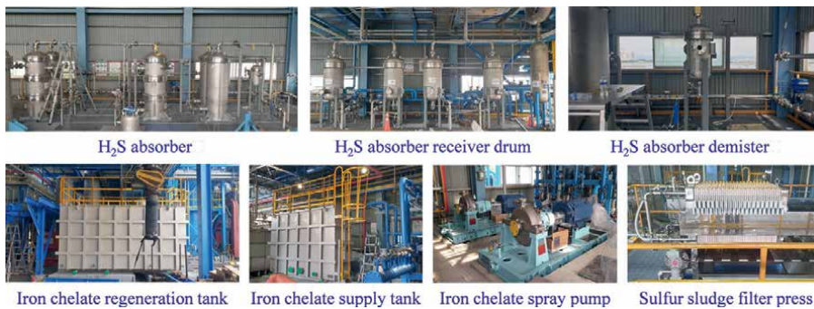
Figure A4. Key components of H_2S removal system (syngas treating capacity 1600 ~ 2500 Nm^3/h ) in demo-scale plant.
