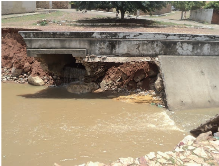
Figure 3. First collapsed storm drain tributary to the Granjeiro stream, the object of this study (The Author, January 30, 2011).
