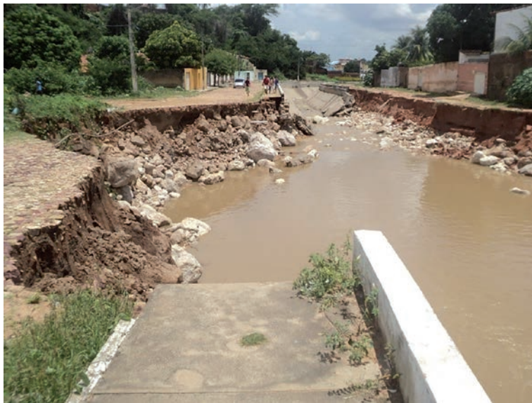
Figure 4. Detailed view of the rupture immediately downstream of the entrance to the first storm drain (The Author, January 30, 2011).
