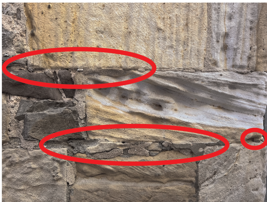
Figure 24. Detail of a sandstone wall in Soria, Spain, where cemented cuttings can be seen (photo by the author).
