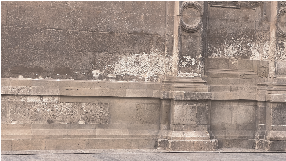
Figure 22. Limestone ashlars with varying degrees of deterioration on the facade of the bell tower of the Cathedral of Murcia (photo by the author).
