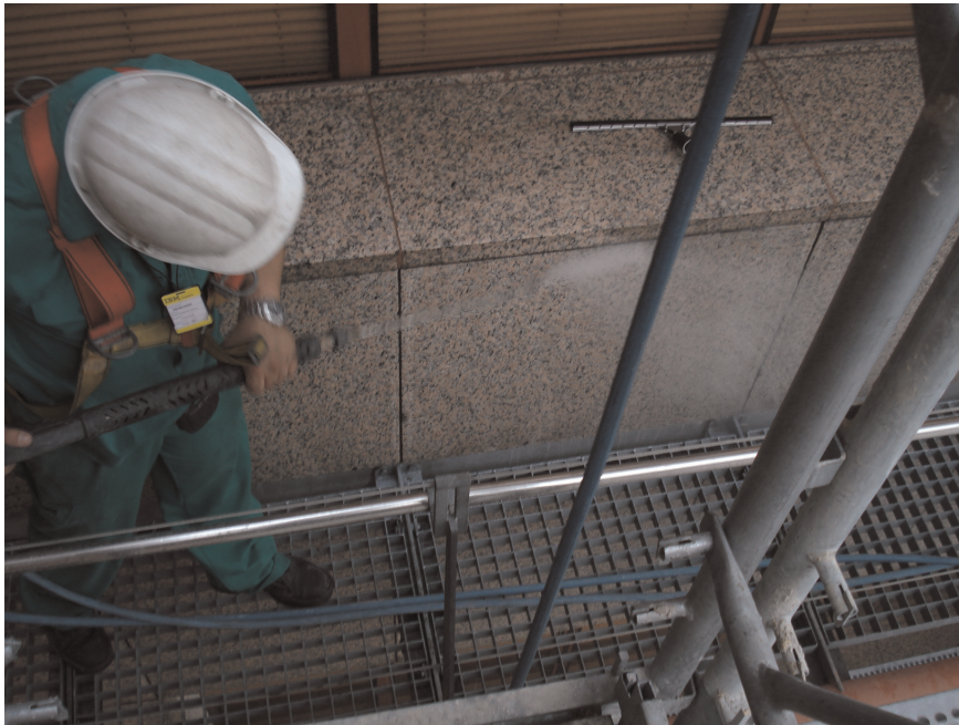
Figure 25. Cleaning operations with water jet and detergent on the pink granite cladding of a building in Madrid (photo by the author).
