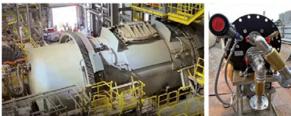
Figure 4. Examples of copper furnace running with oxyfuel and JL flameless oxyfuel burner.
