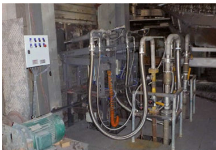
Figure 13. Example of a retractor and burner installation.
