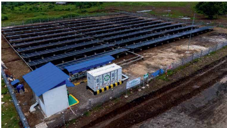
Figure 14. Application of solar PV-BESS technology in Indonesia [29].
