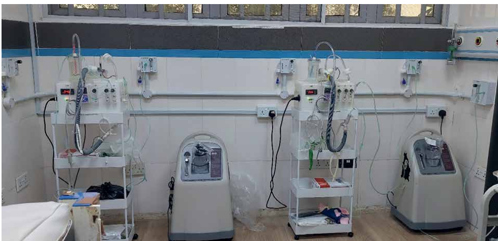
Figure 1. The RespSS corner at the SCBU of the University of Benin Teaching Hospital (UBTH), Nigeria.
